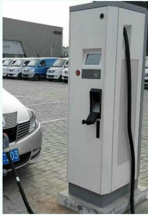
Outdoor (fast charge) charging pile
