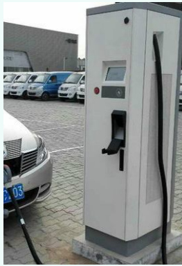
Outdoor charging station
